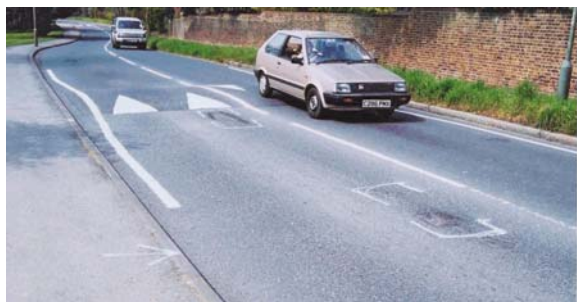
Watts Lane Potholes
